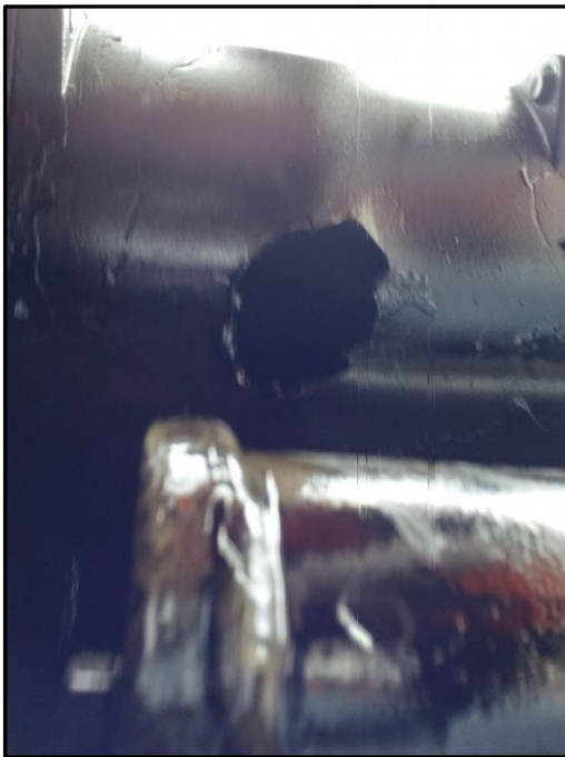
Figure 6. Bottom view of the air intake manifold on locomotive CP 9779, showing the damage and its location (Source: TSB)
