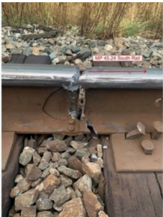
Figure 9. South rail at Mile 45.24, showing that the web and base of the rail are broken (Source: Canadian National)
