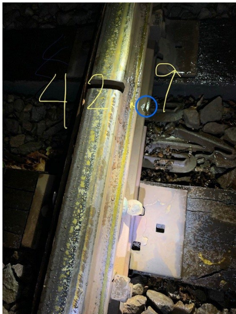
Figure 6. Condition of the track at Mile 42.9, including an impact mark on the gauge side of the joint bar (circled), a shiny mark on the base of the rail, and steel shavings on the gauge side (Source: Canadian Pacific)
