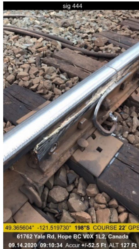
Figure 8. Sheared-off bolt and damaged insulated joint bar at Mile 44.4 of the south rail (Source: Canadian National)
