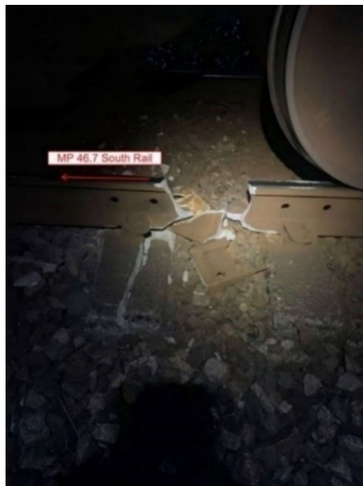
Figure 10. Broken south rail at Mile 46.7, showing a fracture measuring about 4 to 6 inches (Source: Canadian National)
