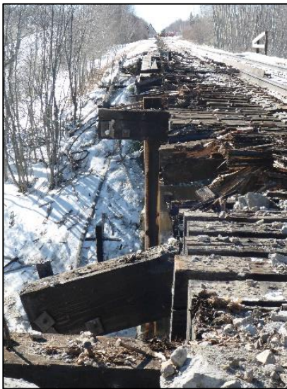
Figure 4. Bridge deck damage (Source: TSB)
