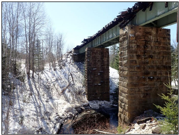
Figure 5. Bridge at Mile 14.9 with damaged ties (Source: TSB)
