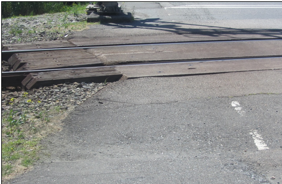
Figure 3. Extension to the crossing surface at the Broadway Street public crossing (Source: TSB)
