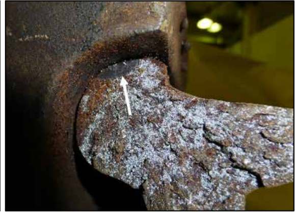
Figure 5. Field-side joint bar with fatigue identified by arrow
