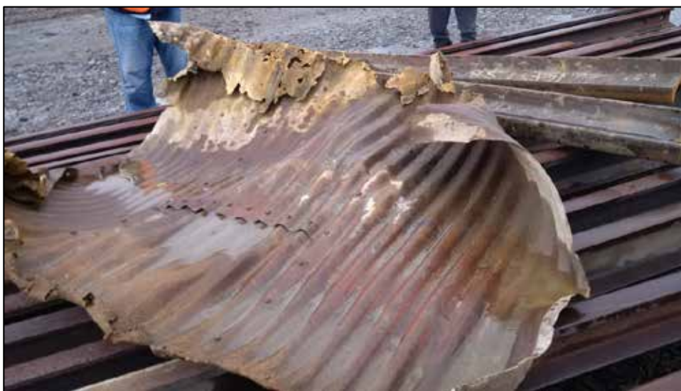
Photo 8. Section of culvert containing rust-through corrosion
