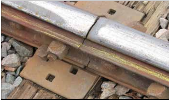
Photo 5. Broken joint bar
