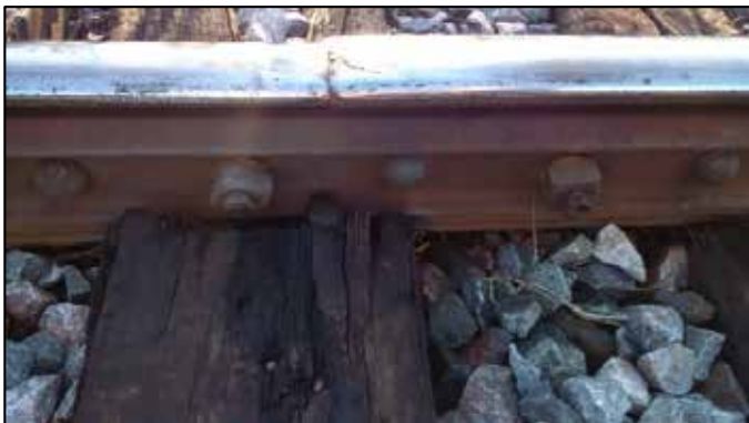
Photo 7. Missing tie plate
