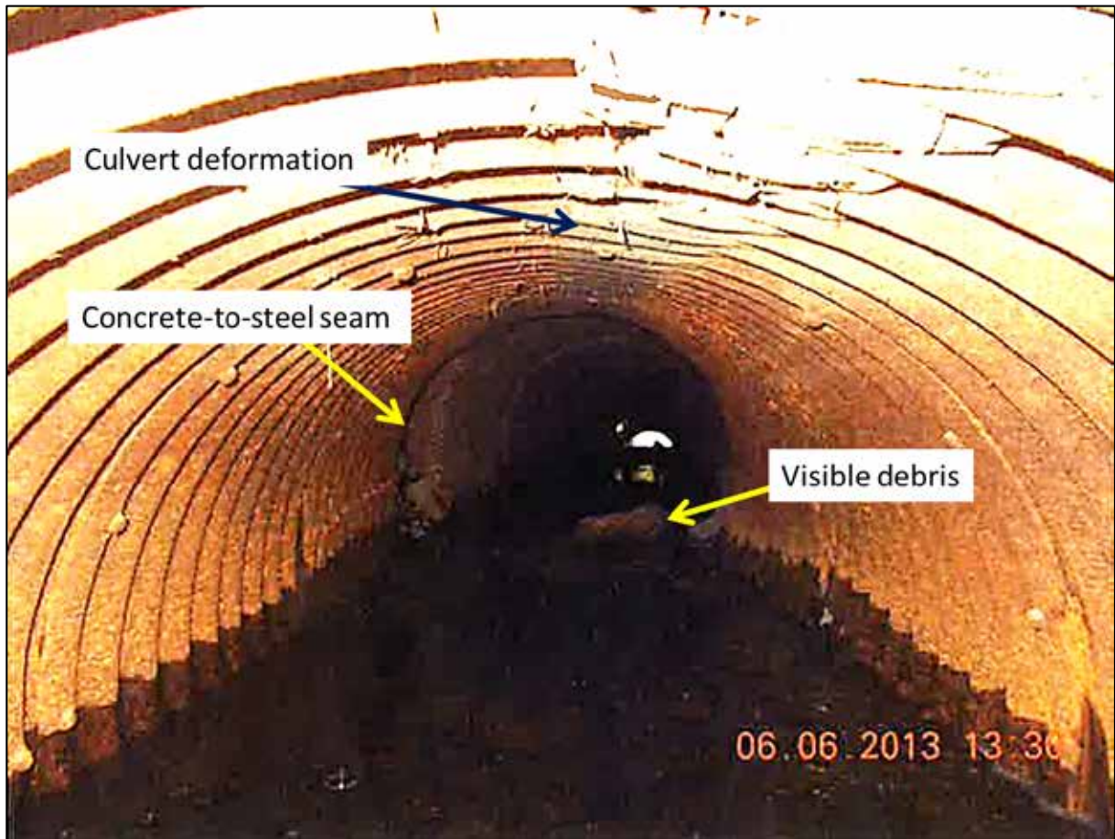
Figure 4. Culvert at Mile 72.08 during June 2013 inspection. Note: brightness adjusted for easier identification of defects. (Source: Huron Central Railway inspection report, with TSB annotations)
