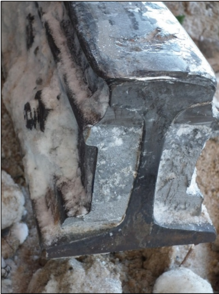
Photo 1. West portion of insulated joint assembly containing broken joint bars and intact rail recovered from the site
