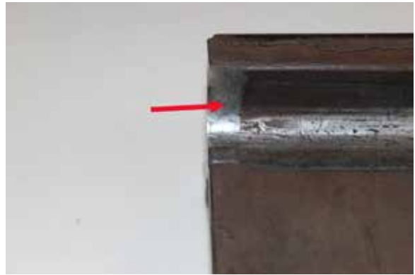
Photo 9. Rubbing or fretting mark on the fillet under the rail head
