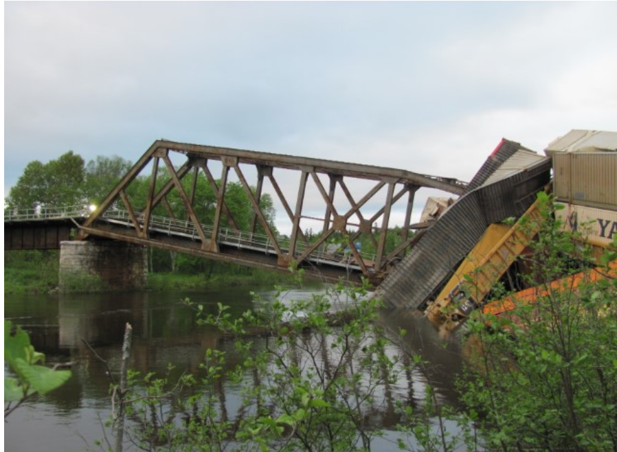
Photo 1. Collapsed south end of the railway bridge
