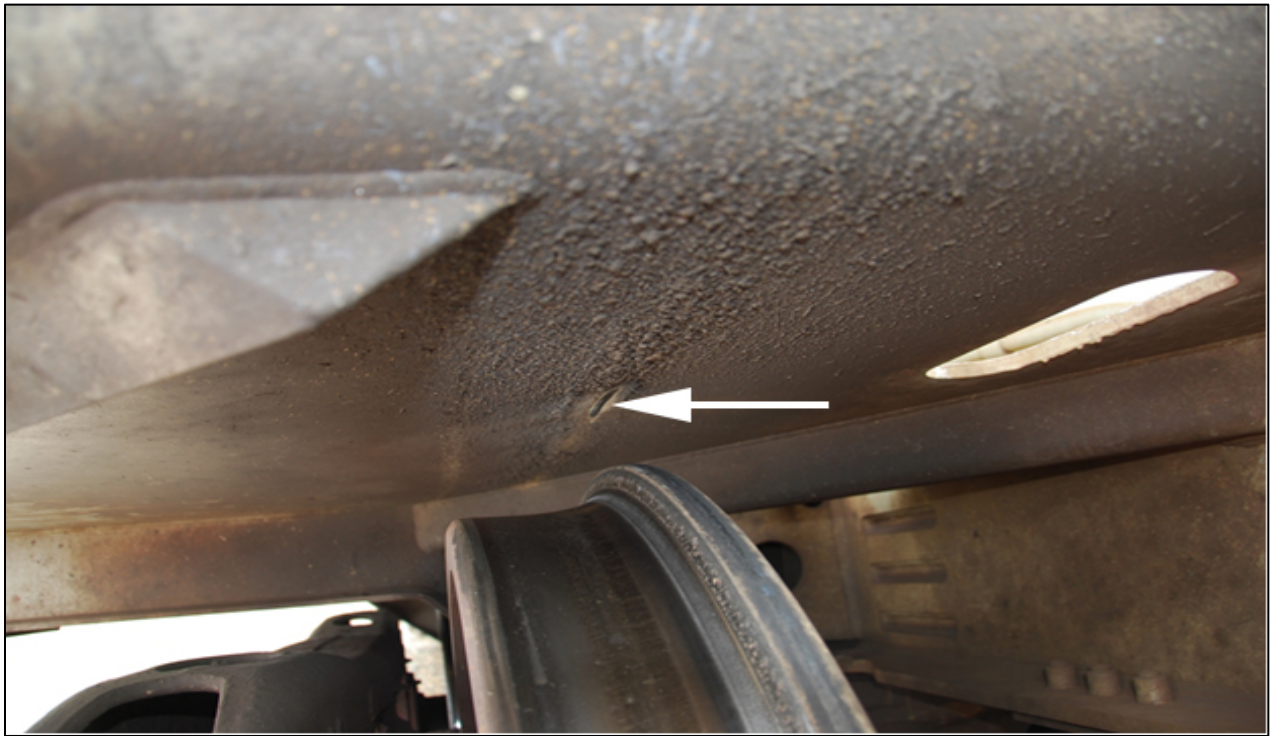
Photo 3. Impact marks where the wheel struck the deck plate
