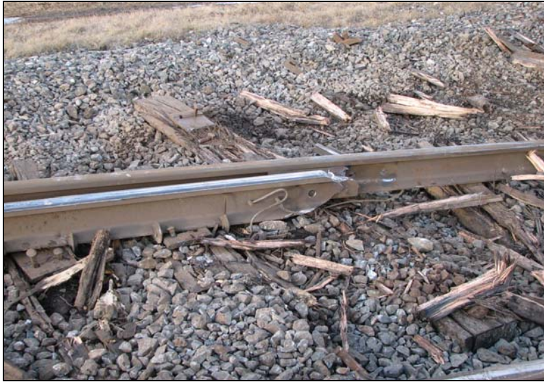
Photo 1. Track ties beneath the heel block joint
