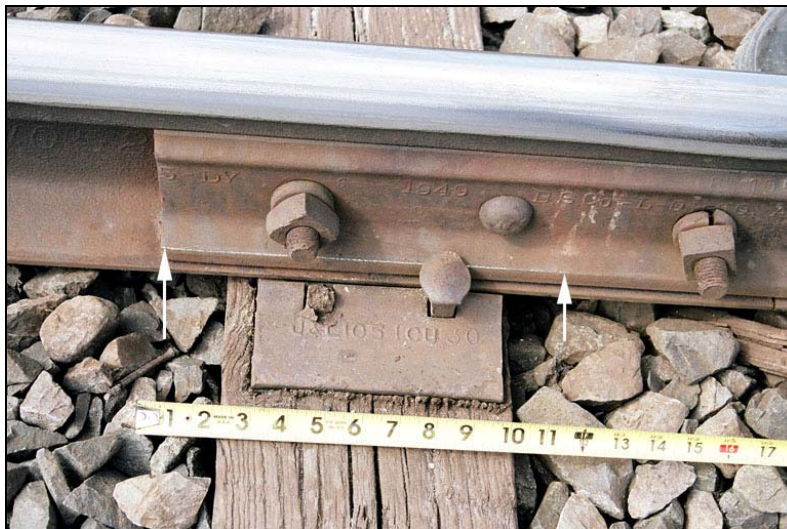
Photo 2. Rail creep marks observed along the base of a joint bar
