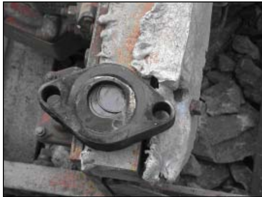
Photo 6. Defective locomotive one-way check valve
