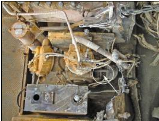
Photo 5. Broken pressure cylinder on the two-stage air compressor
