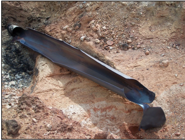
Photo 4. Failed section of the Westcoast Nig Creek pipeline
