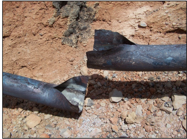
Photo 5. Failed Bonavista pipeline
