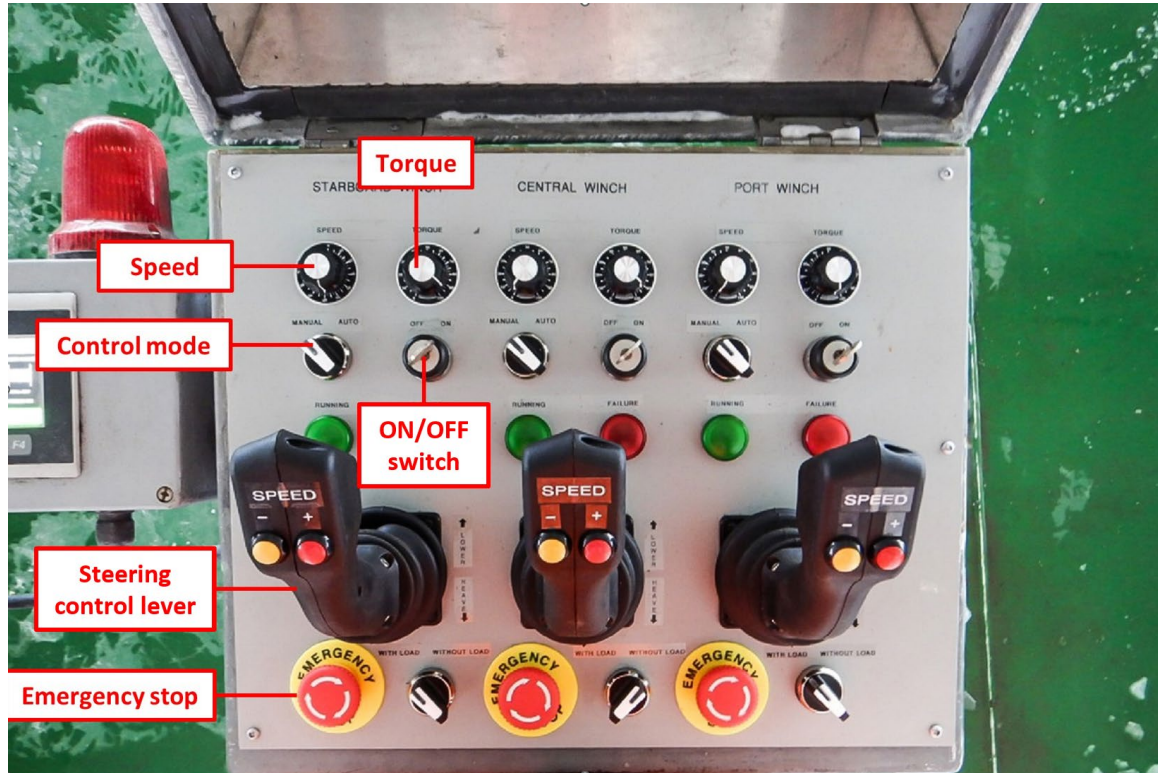
Figure 7. Main control unit (Source: TSB)
