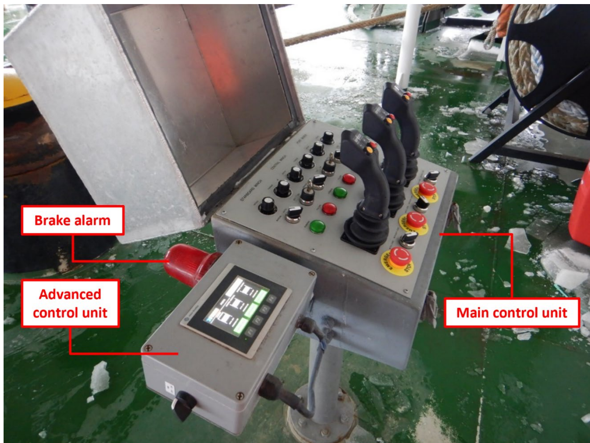
Figure 6. Overview of aft mooring winch control station (Source: TSB)
