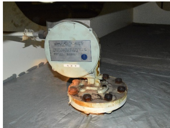
Figure 14. Type of float level indicator that was originally fitted over the opening of the sounding pipe for the settling and service tanks (Source: TSB)
