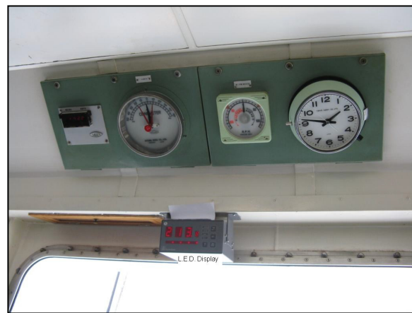
Photo 4. LED analogue repeater and rudder angle indicator.
