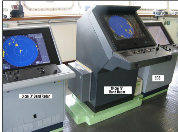
Photo 3. 3 cm radar, 10 cm radar and ECS.
