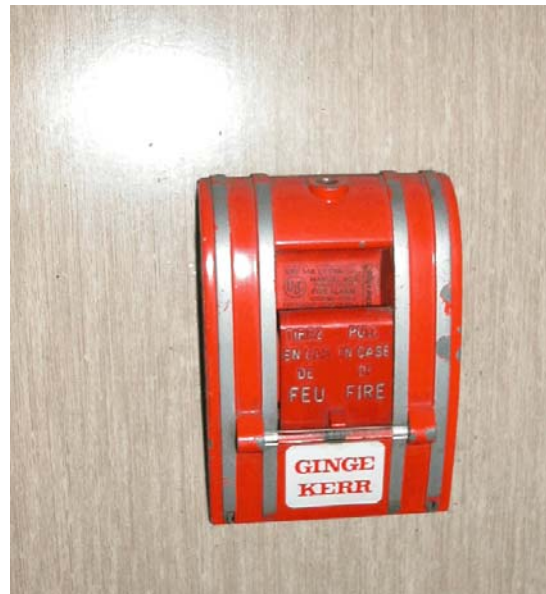
Photo 4. Typical manual pull station
