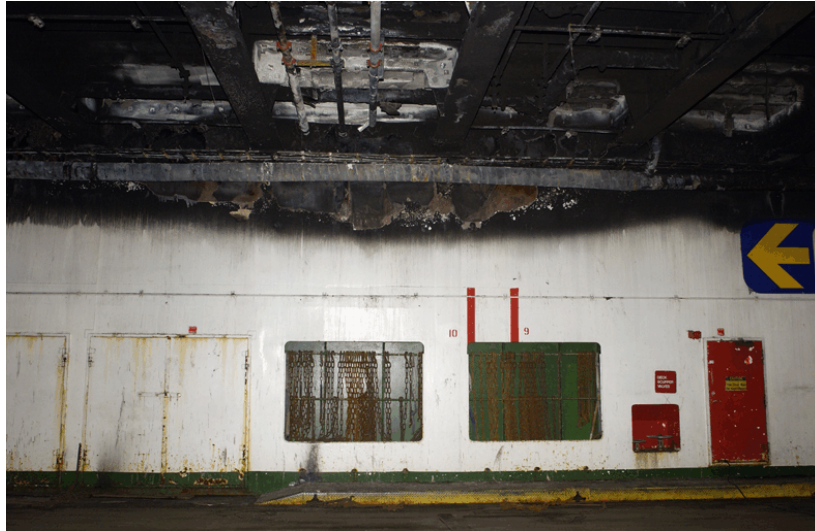
Photo 2. Damage to deckhead
