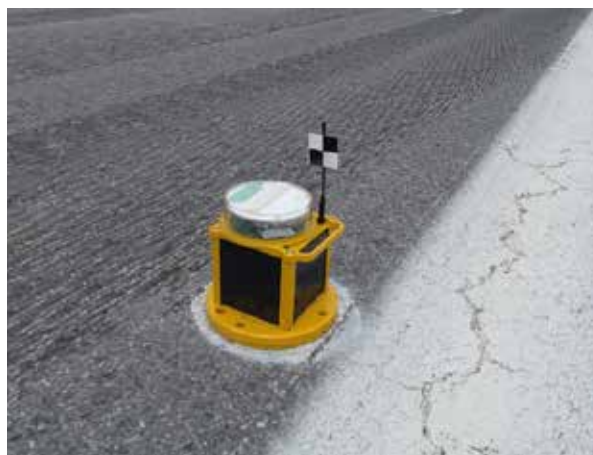
Figure 5. Temporary runway edge light
