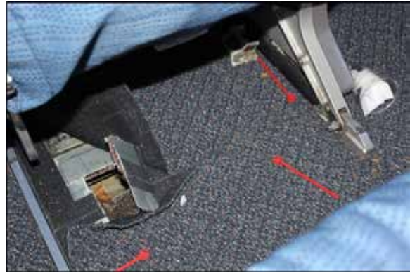
Figure 11. Floor damage forward of passenger seat 33D
