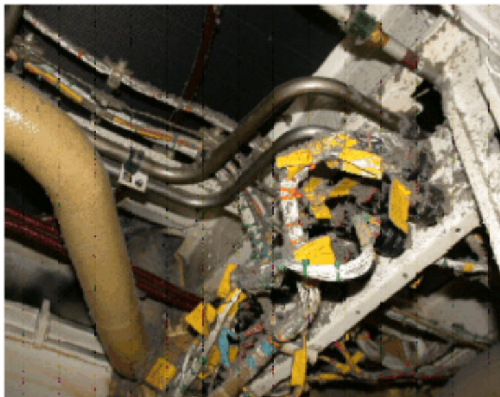
Photo 6. Dust and lint accumulation on wiring bundles behind wall panel
