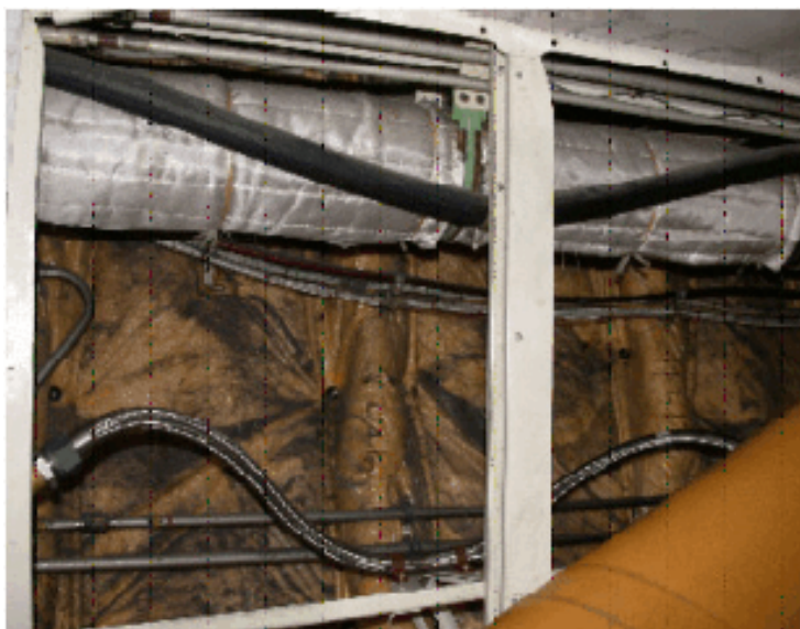
Photo 7. Dust and lint accumulation on thermal acoustic insulation behind wall panel
