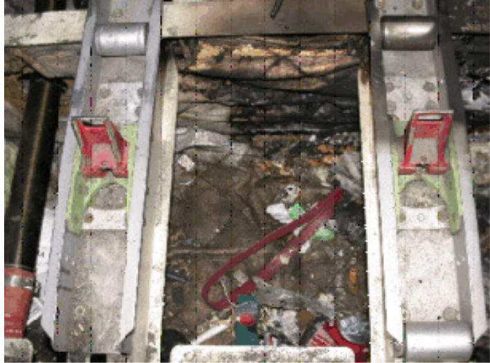
Photo 4. Contaminated insulation blankets and debris
