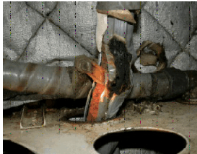
Photo 5. Burned heater ribbon behind aft wall
