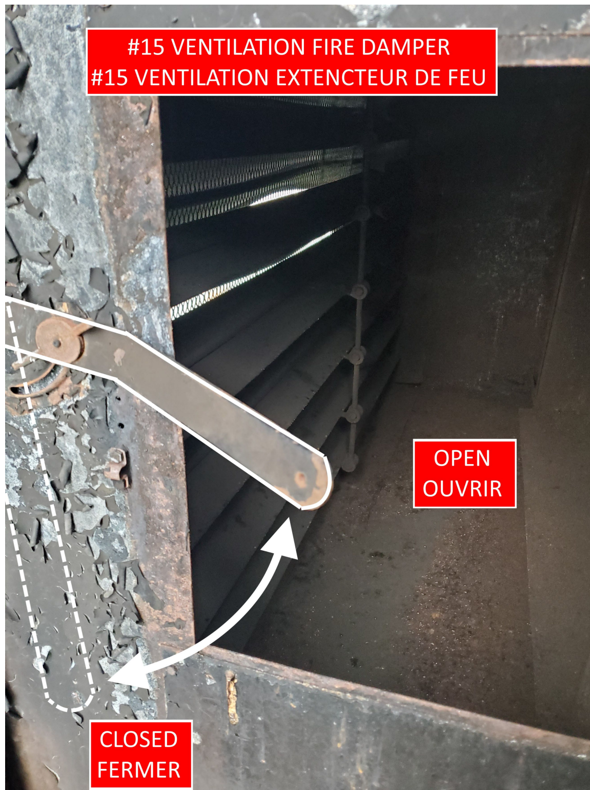
Figure 13. Vent 15, with the damper handle in the open position and an access panel removed. The labels represent the location and appearance of the identification placards that were destroyed by the fire. (Source: TSB)
