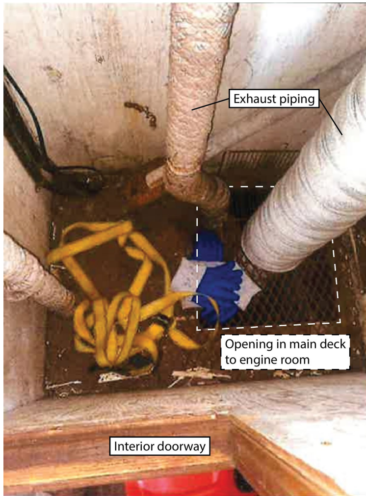
Figure 3. Photo of exhaust trunking taken in 2020 (Source: Third party, with TSB annotations)
