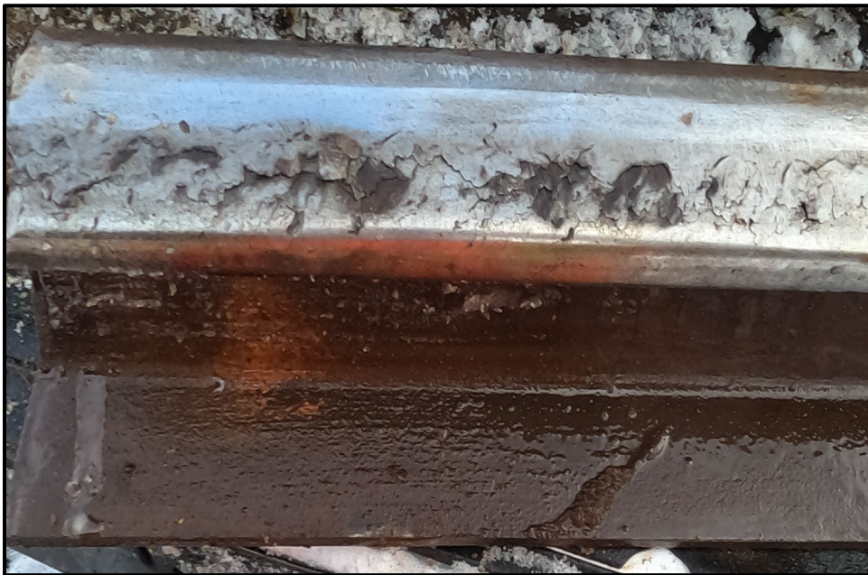
Figure 3. Recovered broken rail with head checking (Source: TSB)
