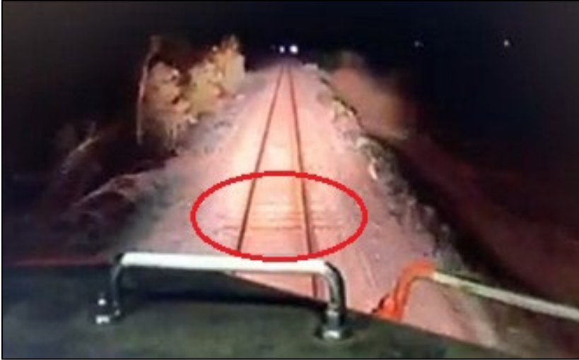
Figure 6. Still image captured from the forward-facing video camera on the head-end locomotive showing the location where the locomotive dipped slightly to the right on the west rail (circled) (Source: Canadian Pacific Railway Company)
