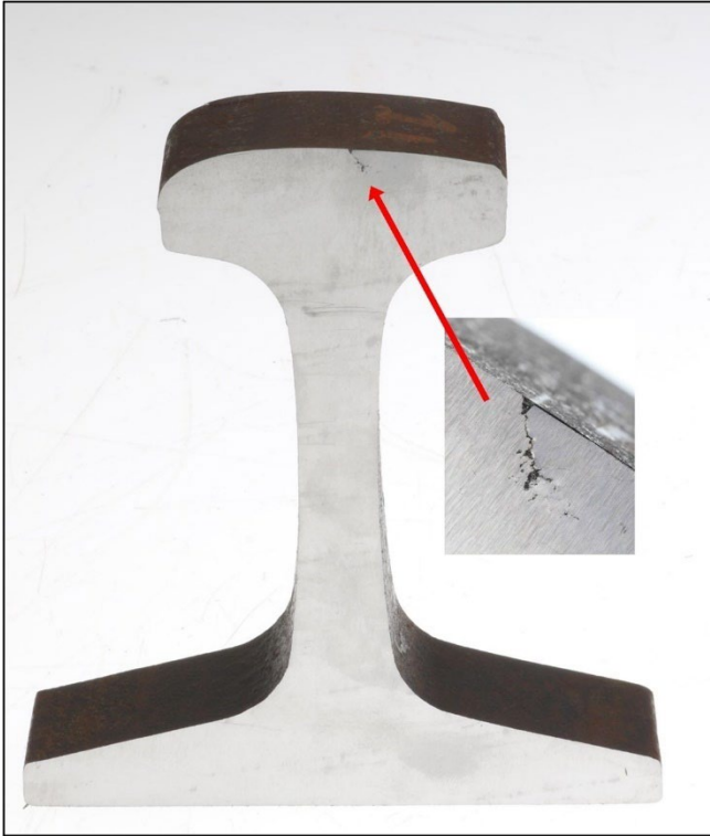
Figure 9. Rail 1 cross-section showing the crack (Source: TSB)
