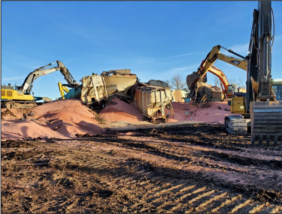
Figure 3. Site remediation activities for released potash (Source: TSB)
