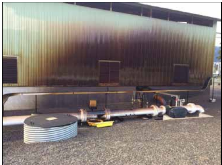
Figure 2. Oil spray on the side of the pump building (Source: Trans Mountain)
