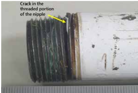
Figure 3. Crack in the ¾-inch threaded portion of the nipple (Source: Trans Mountain, with TSB annotations)
