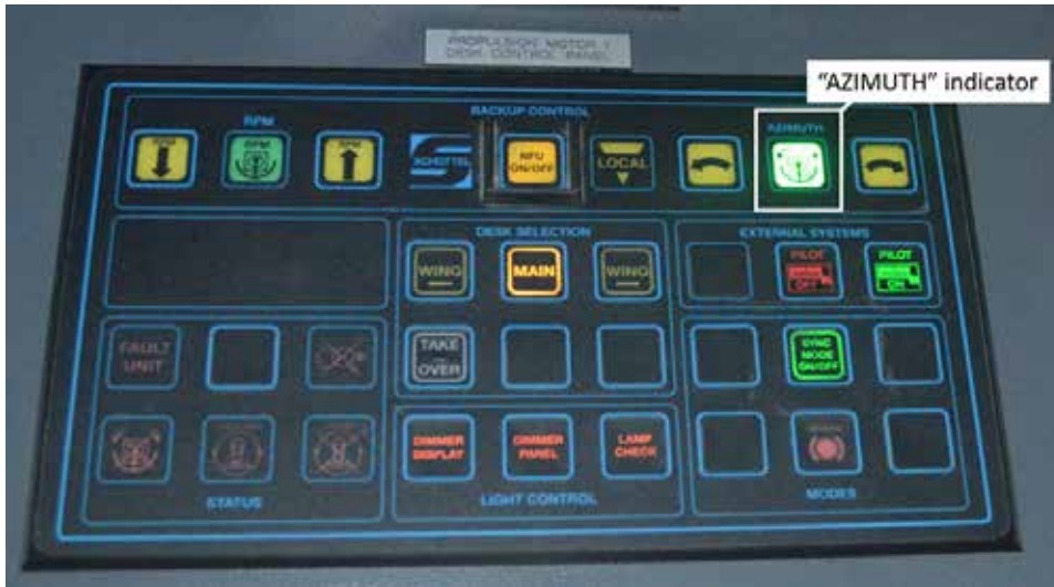
Figure 4. Location of the “AZIMUTH” indicator on the propulsion control panel
