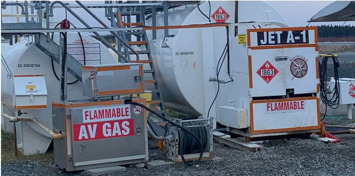
Figure 1. Fuel storage tanks at Pickle Lake Airport (Source: North Star Air Ltd., with permission)
