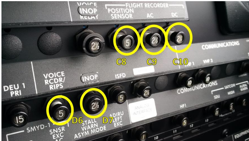
Figure 3. Occurrence aircraft panel with correct cockpit voice recorder and flight data recorder circuit breakers disabled (Source: TSB)
