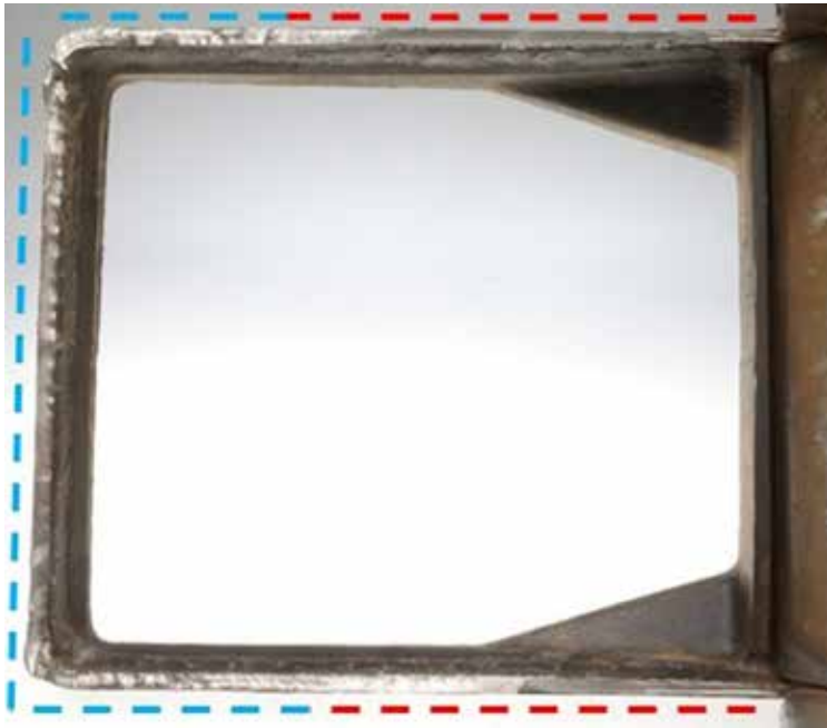
Figure 5. Fracture surface in the welded region joining the crane column and the crane base. Note the flat region (outlined by blue dashes) and the angled region (outlined by red dashes).
