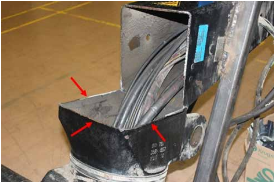
Figure 3. Location of the failure of the crane column weld, indicated by the red arrows
